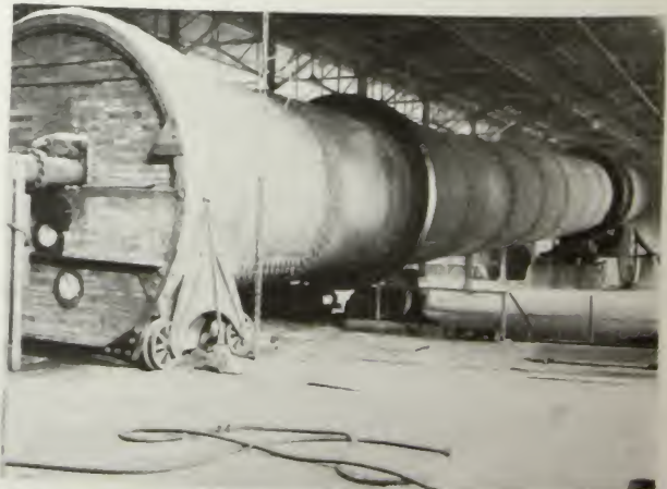
A modern rotary cement kiln in which the raw materials are burned to clinker.
